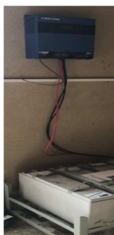
Figure 2: installed Electricity-grid charging system
