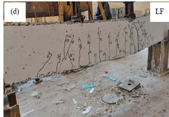
Figure 17: Crack patterns and failure shapes of lightweight concrete with GFRP
