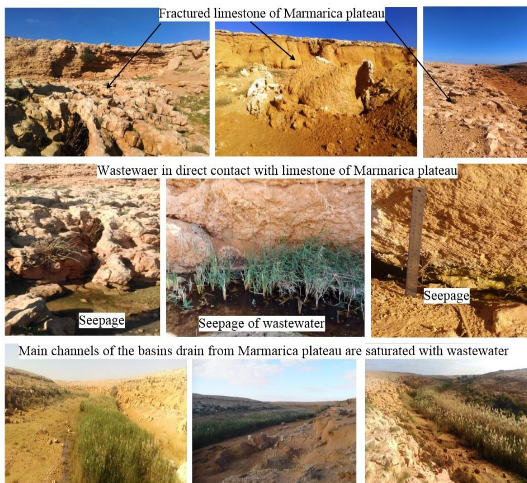
Fig. 4. Field photos show the effect of wastewater on plateau rocks where they are in a direct contact.
