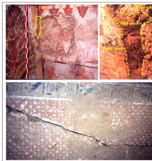
Figure 1. (Up) Stratigraphic structure of a wall painting, example from the Theban tomb TT278, (Bottom) wide crack and structural defects of the ceiling, Theban tomb TT192.
