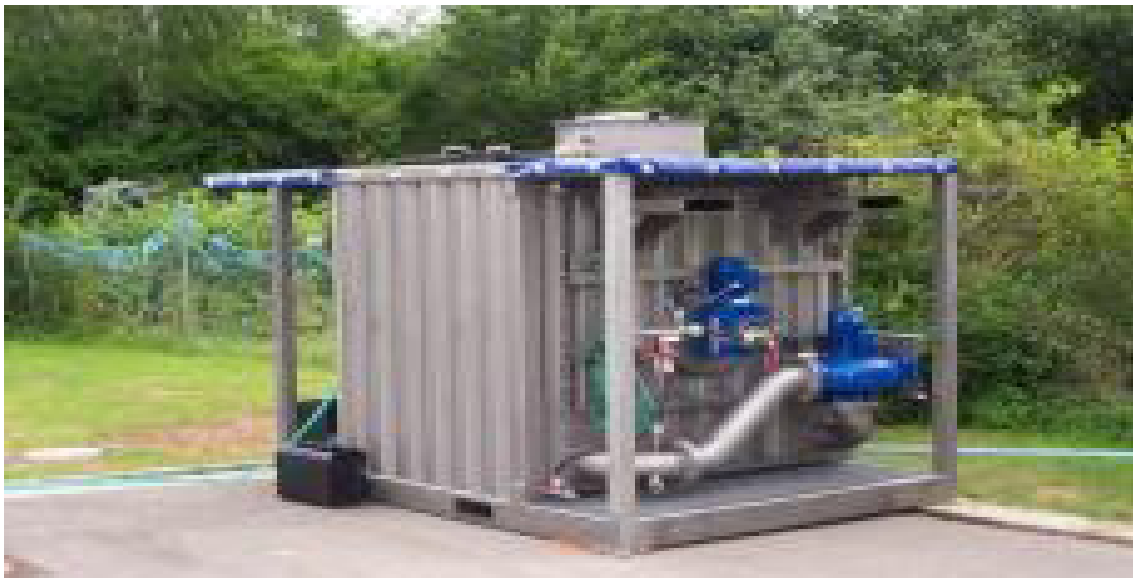
Fig. 10. illustration of MBR compact system for municipal wastewater treatment in Zenien Sewage Treatment Plant, Cairo, Egypt..
